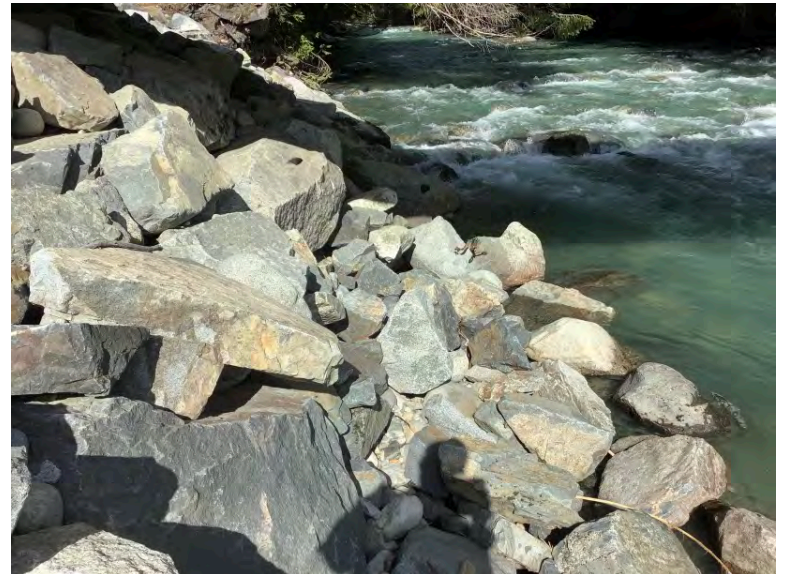
Right Bank Abutment when facing downstream - riprap unravelling a bit
